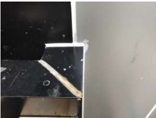
Figure 5: 8mm hole above parapet feature
