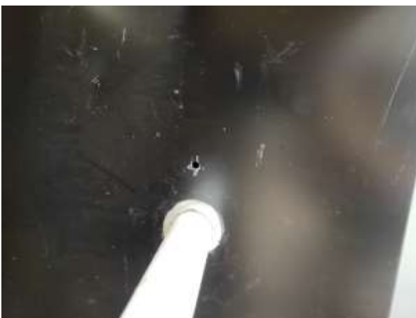
Figure 7: 8mm hole above pipe penetration
