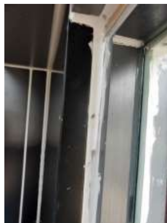
Figure 8: 8mm hole at 3/4 window height in caulking
