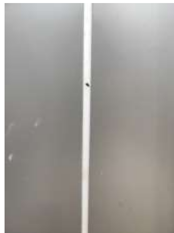
Figure 6: 8mm hole in panel joint caulking
